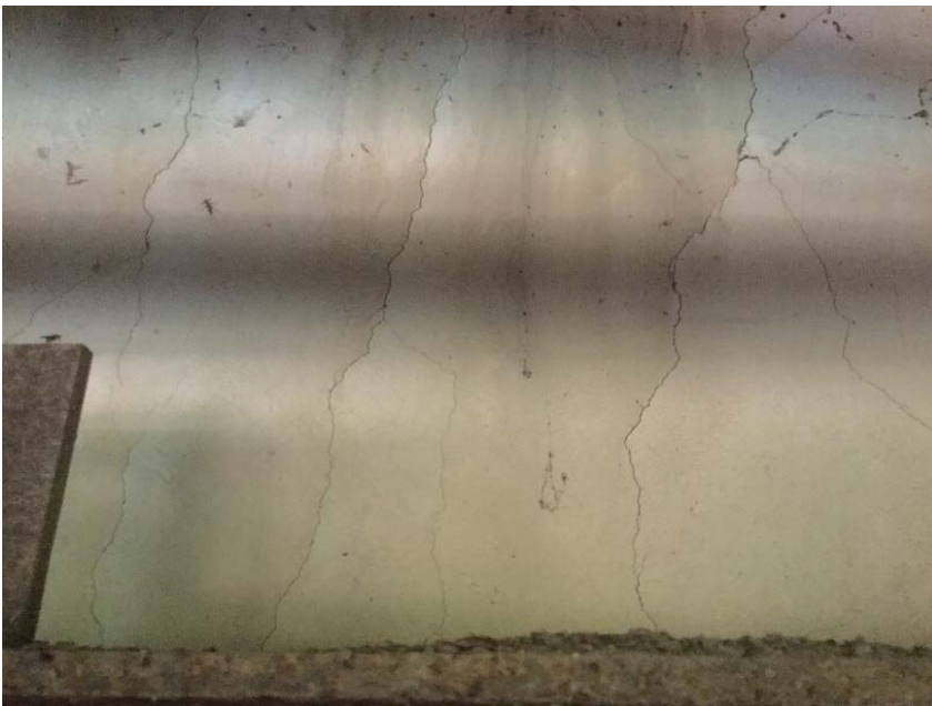
Right bank ballast wall cracks
